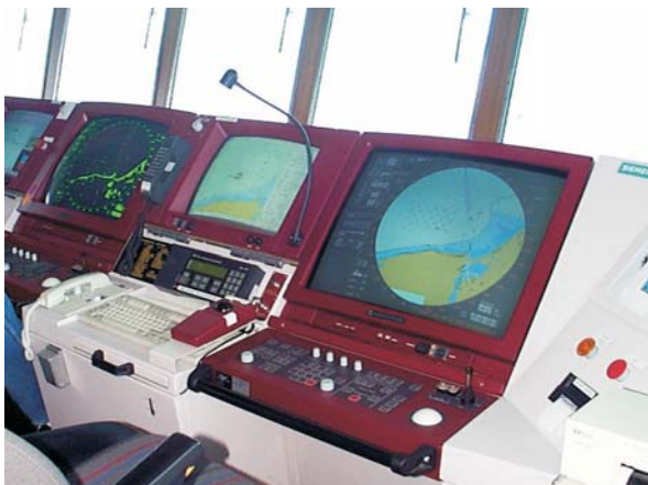
Fig. 3. ECDIS installation in the ship (URL 5)
